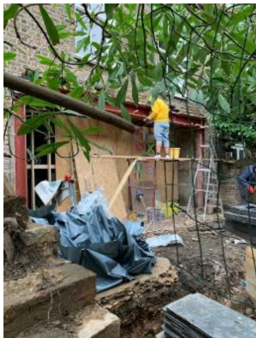
Photo of rear elevation (from neighbour, showing lower ground floor works dated 2 Nov 2022)
